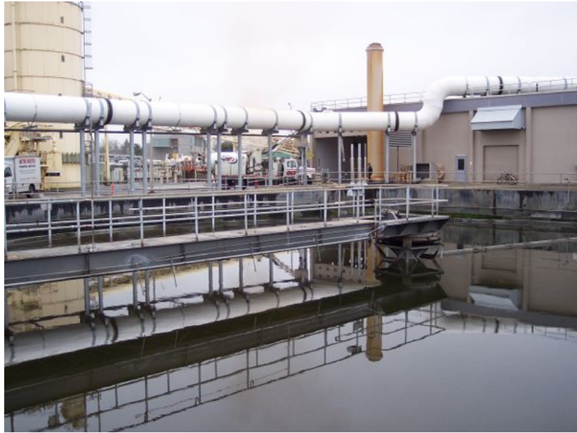
Primary treatment tanks in Oregon, USA.
