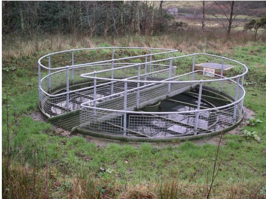
Secondary clarifier at a rural treatment plant.
